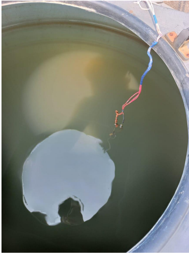
Fig.3. (a) Sensor inside the overhead tank
