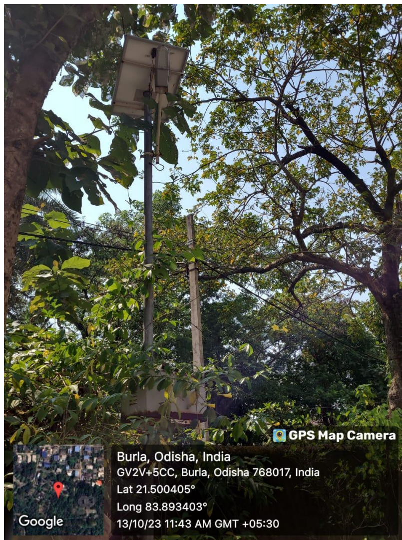
Fig.1(a). Solar street lamp in residential campus
