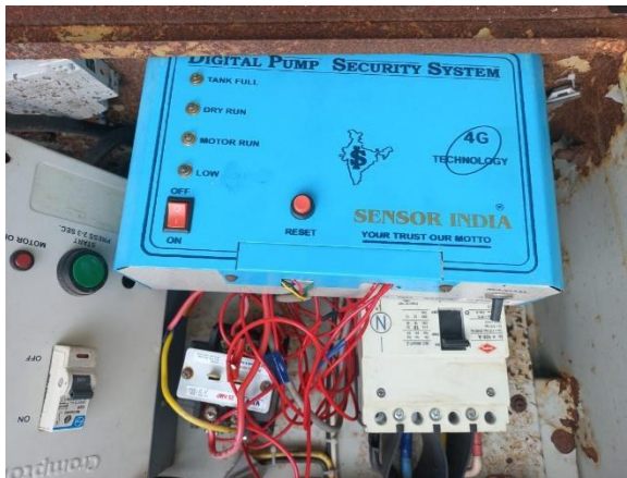
Fig.3. (b) Control Circuit in the pump house
